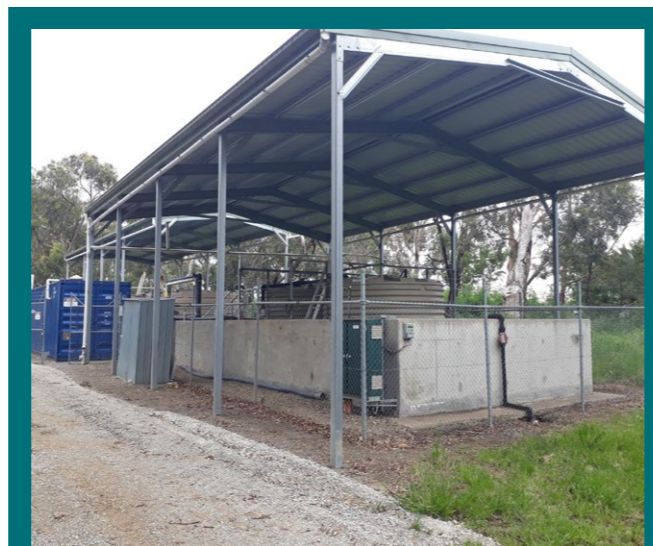
Coldstream leachate plant – the plant processes leachate liquid collected from the landfill for disposal into the sewer system. This is important to ensure that the liquid does not contaminate local groundwater and the surrounding environment.
